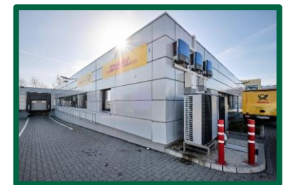
Heat pumps in our ~150 carbon-neutral buildings
